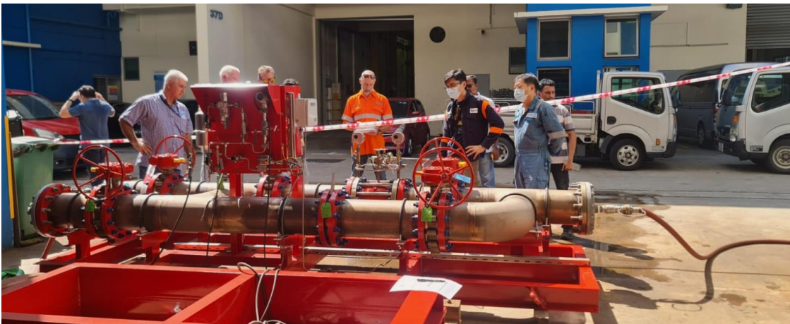
Testing of Wilsafe Deluge Skid with offshore customer and classification society
