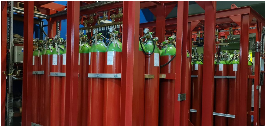
Wilsafe delivery of Clean Agent System (Inergen)
