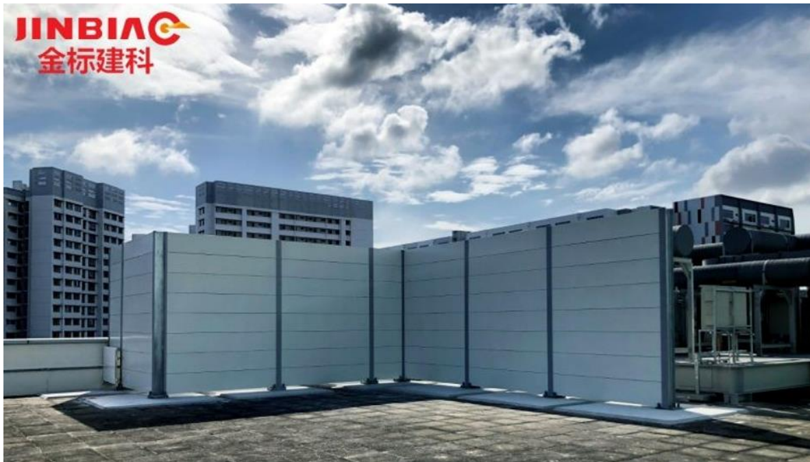
Hebei Jinbiao's permanent noise control barrier for an industrial building
